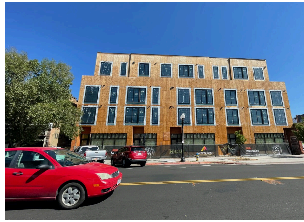
Construction of a five-story apartment building on Historic 25th Street in Ogden has been on hold since late March due to use of wood framing that is insufficiently fireproof, according to city officials.
